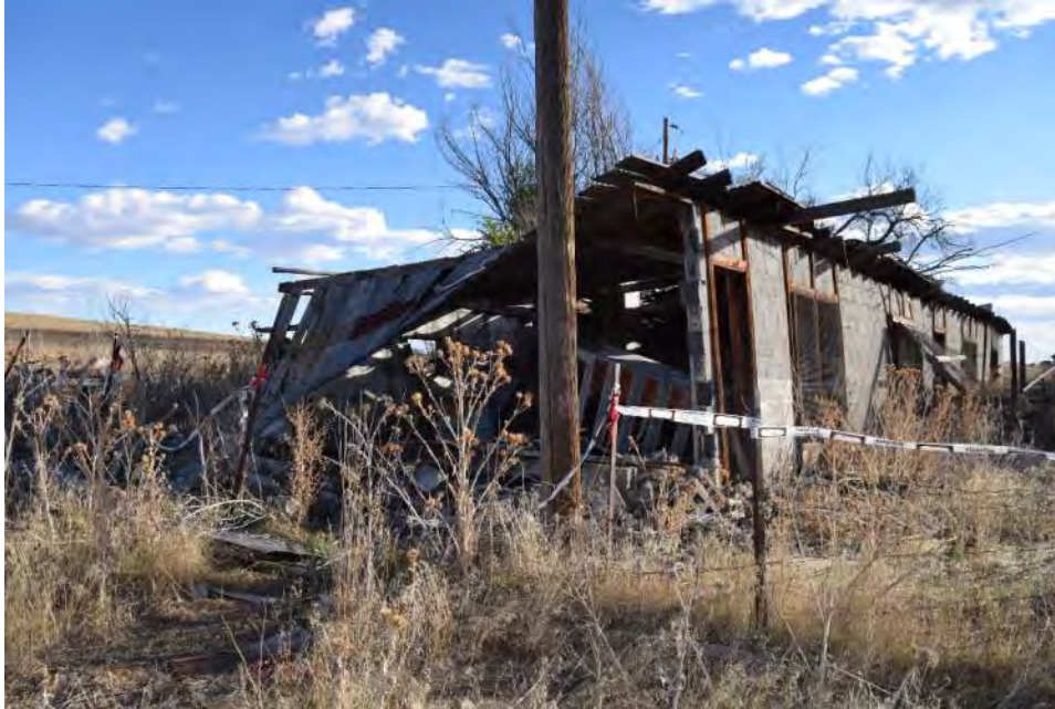
Figure 6. Collapsed west wall of Outbuilding #1.
