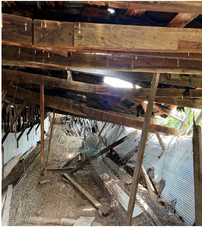
Description: Structure 6, ACM Roofing Tar Paper Debris 7/15/24 Inspection
