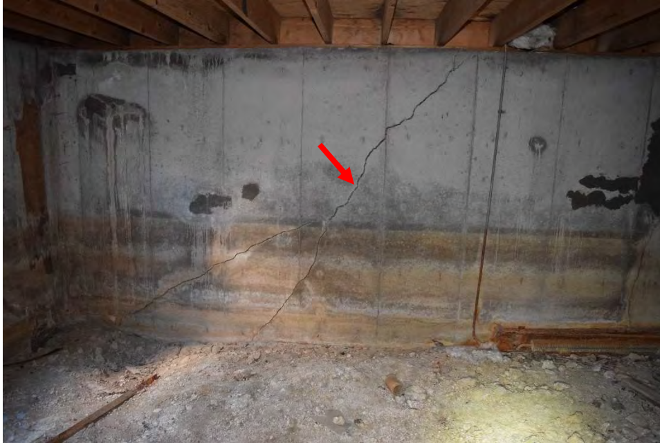
Figure 6. Large crack in the wall of the underground basement at the Original Farmhouse.
