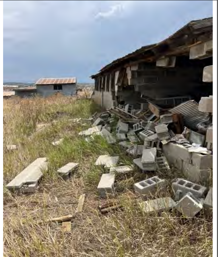
Description: Structure 7, ACM CMU Patch Tar 7/15/24 Inspection
