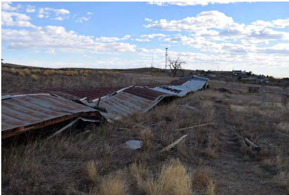
Figure 19. Multiple partial collapses of the Hen House roof.
