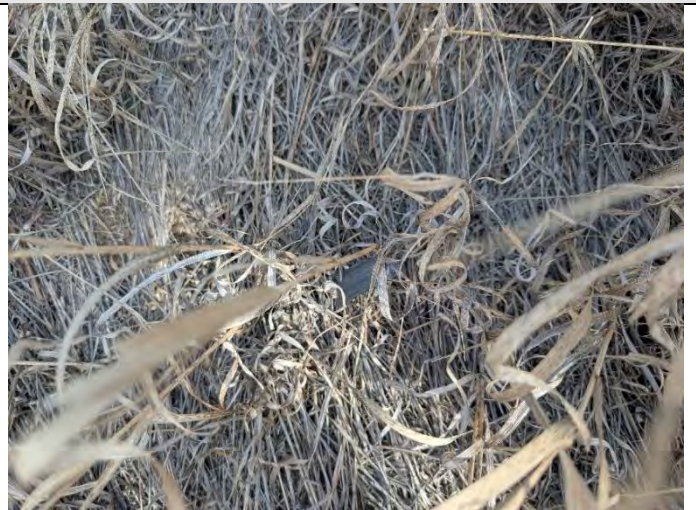
Description: Structure 5 Debris 9/9/25 Inspection
