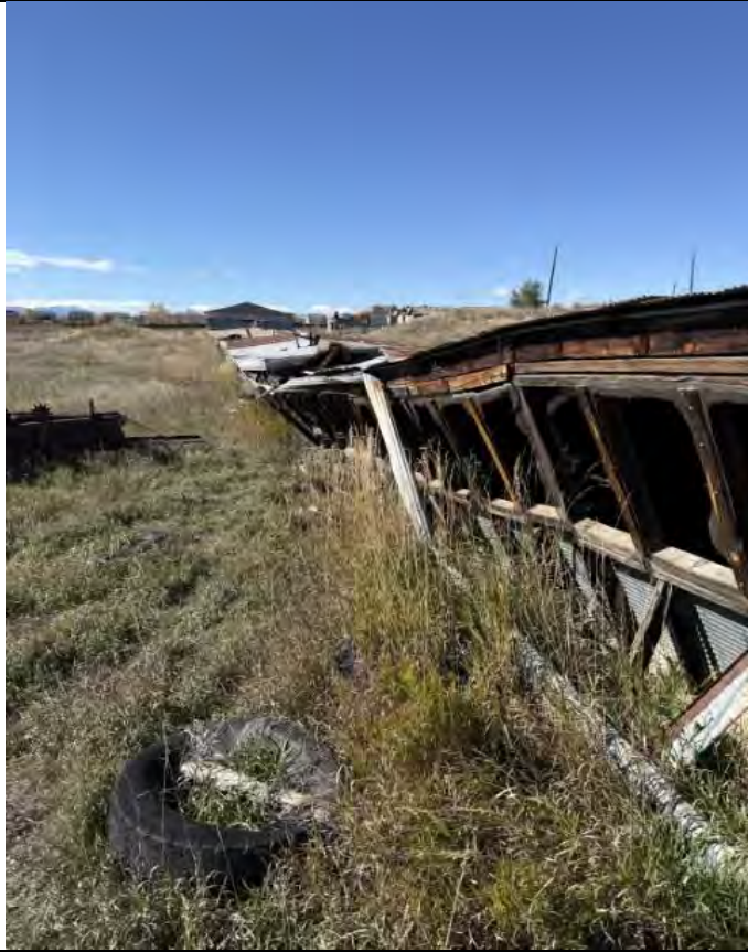
Description: Structure 6, east view, south side, visible lean to the structure, area of slow active collapse
