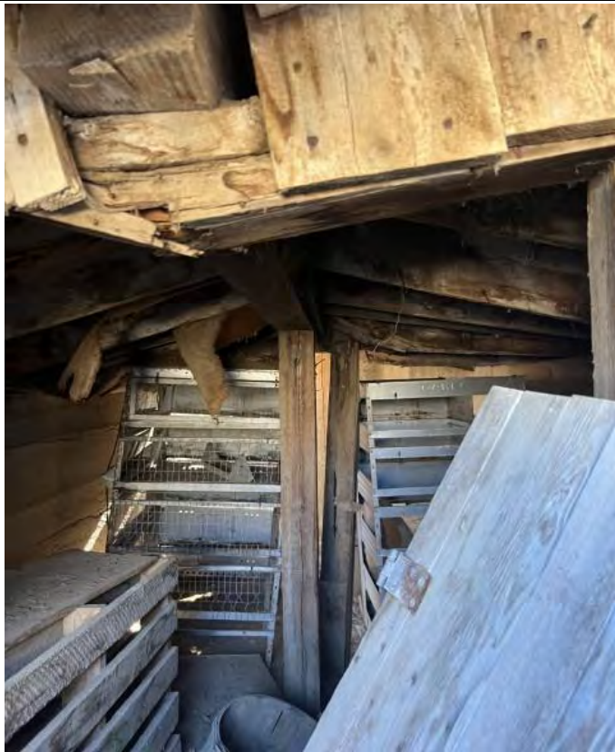
Description: Structure 6, ACM Roofing Tar Paper 7/15/24 Inspection (Prior to Cave-In)
