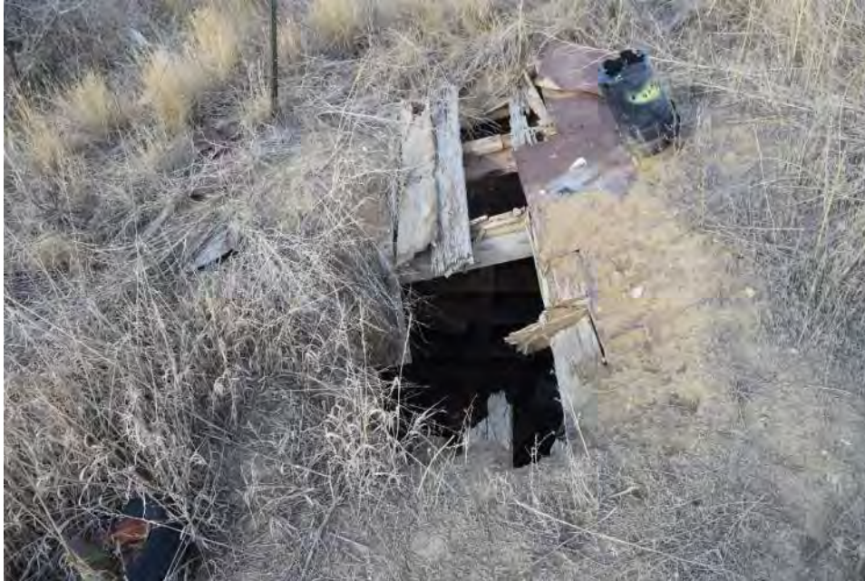
Figure 22. A cave in of the Cellar on the west side.
