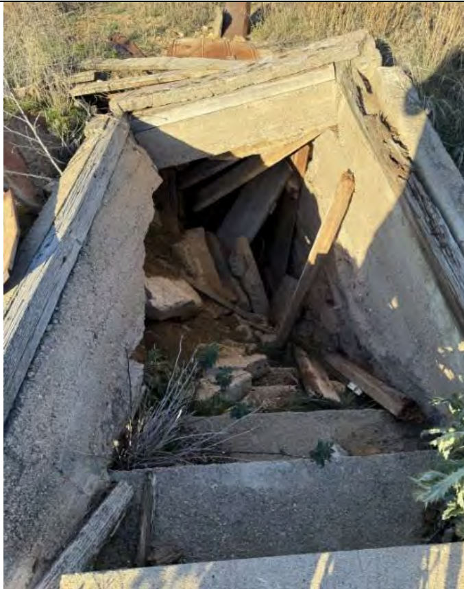
Description: Structure 3, entry stairs blocked by cave-in
