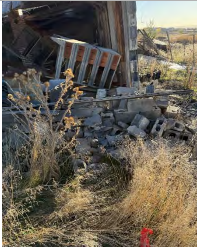
Description: Structure 5, west side collapse & debris
