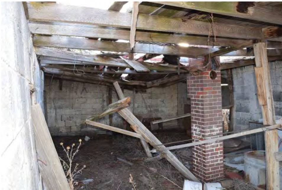
Figure 7. The east half of the roof of Outbuilding #1 beginning to collapse.
