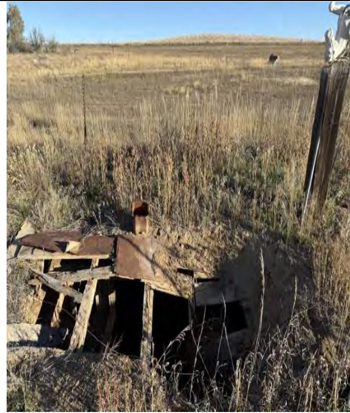
Description: Structure 3, center vent area collapse
