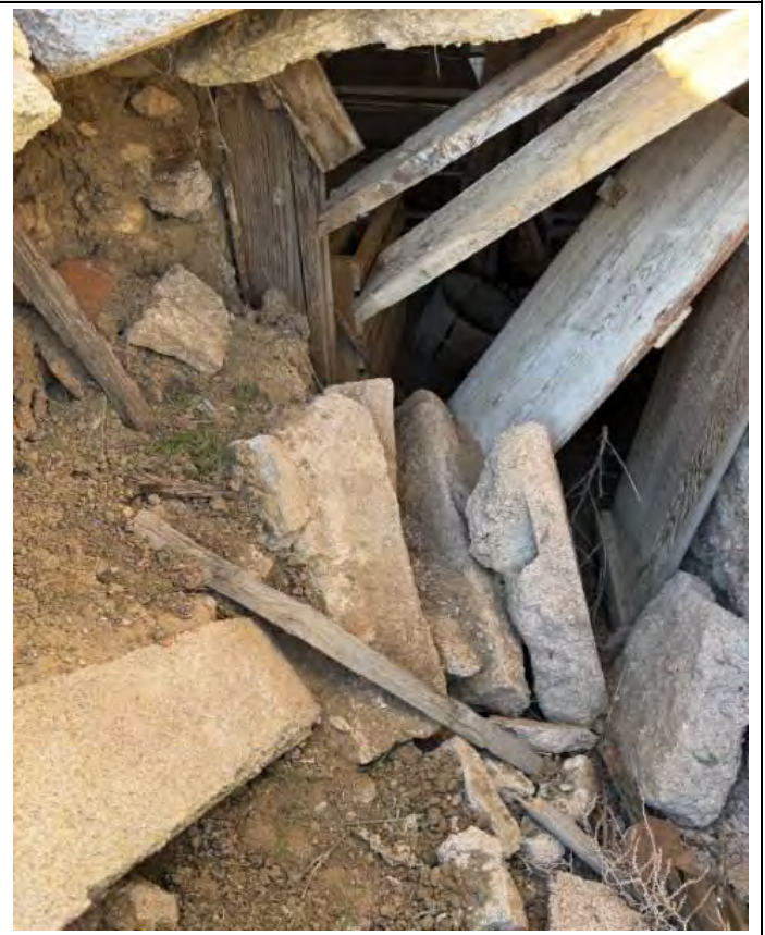
Description: Structure 3, center vent area entry stairs wall collapse
