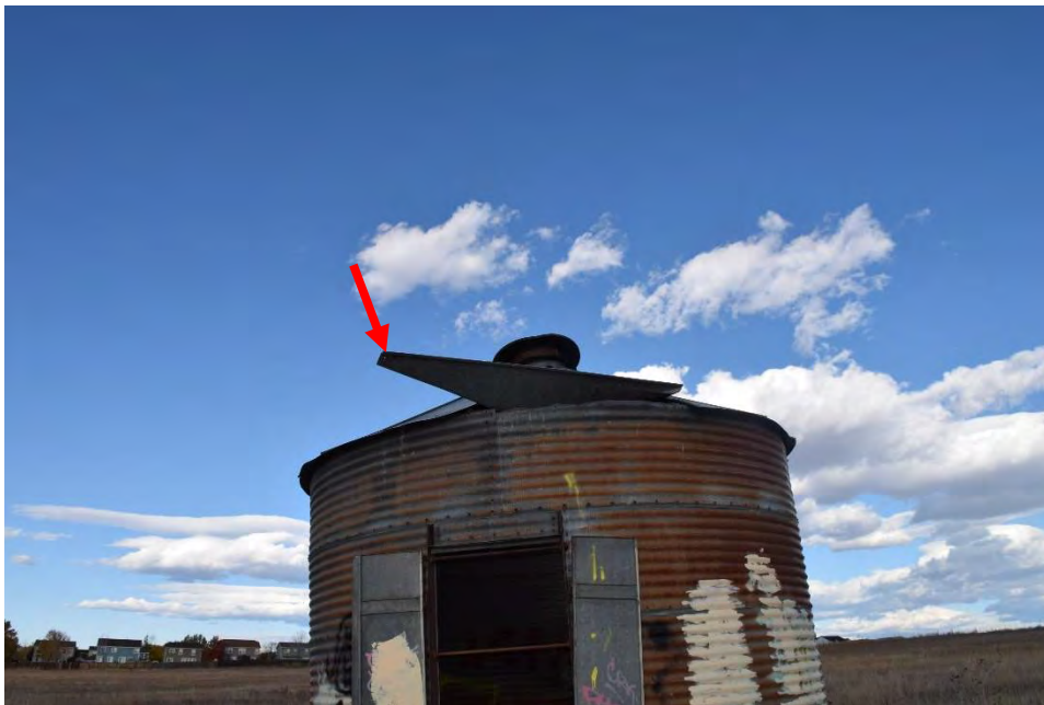
Figure 17. Displaced metal roof panel sitting atop the Silo.
