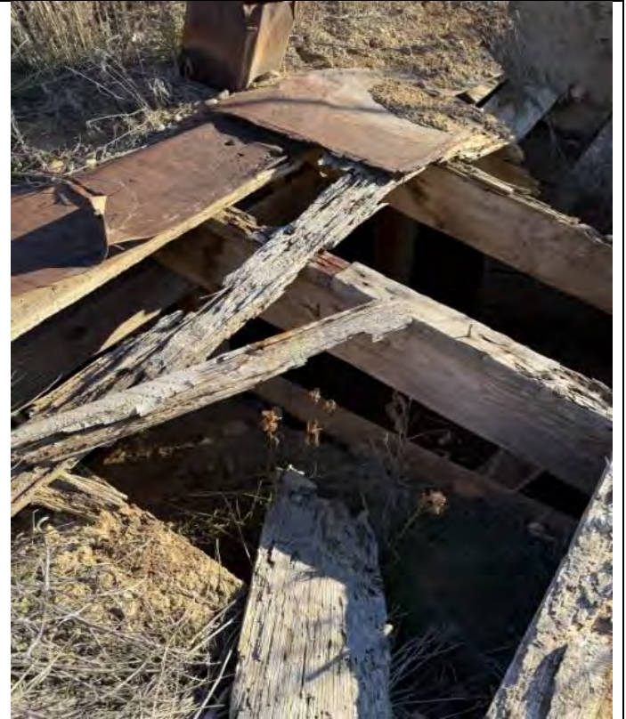
Description: Structure 3, center vent area collapse
