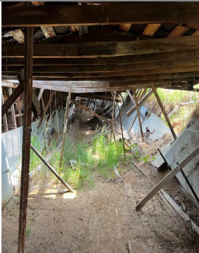
Description: Structure 6, ACM Roofing Tar Paper Debris 7/15/24 Inspection
