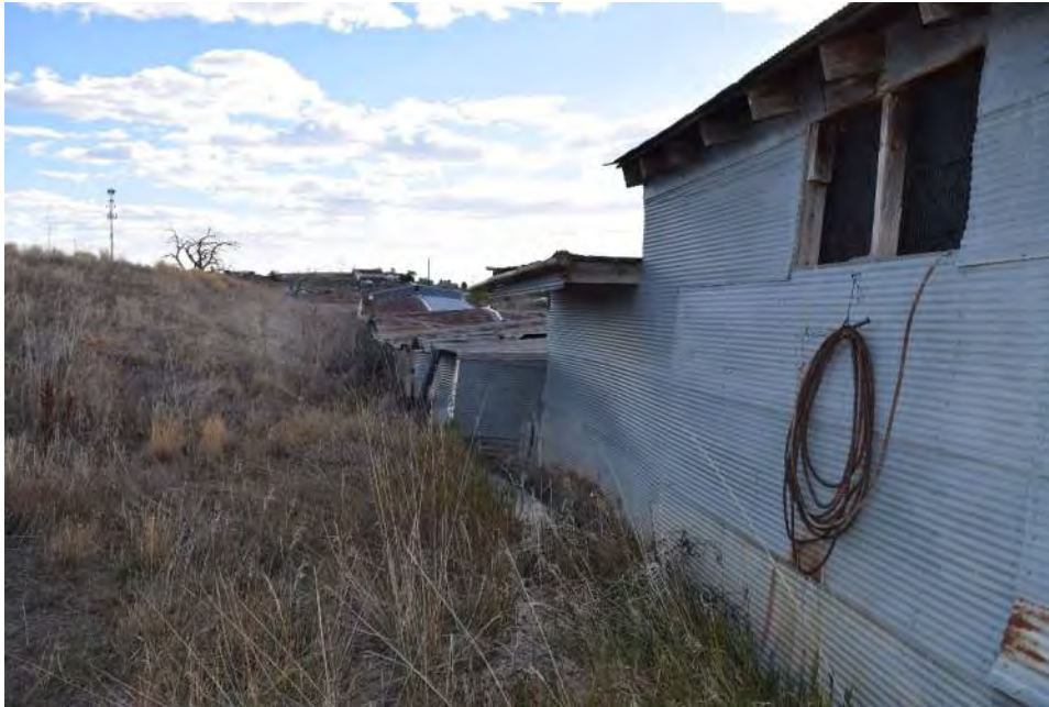
Figure 18. The north wall of the Hen House beginning to bow inwards.
