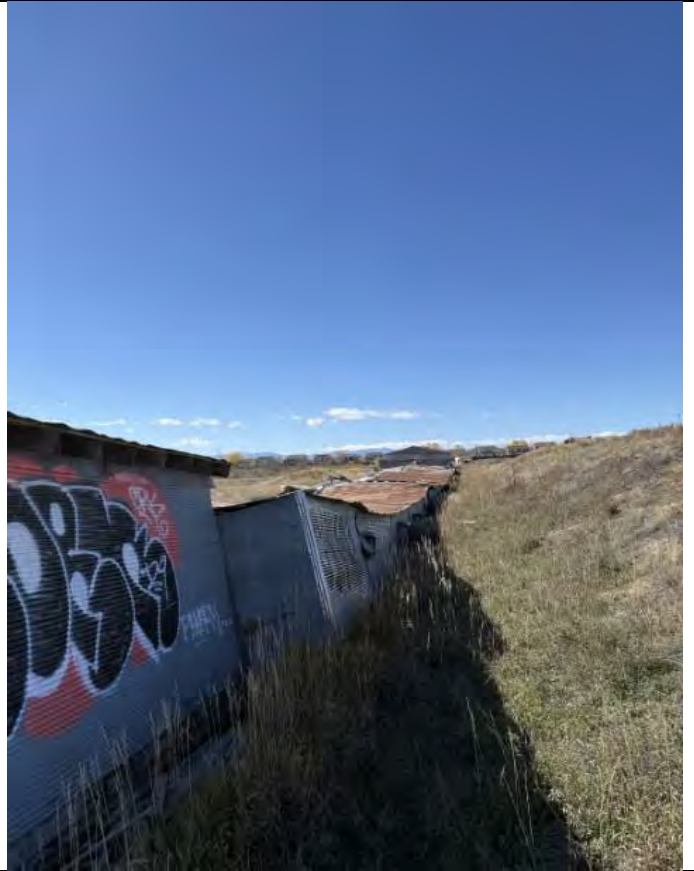
Description: Structure 6, east view, south side, visible lean to the structure
