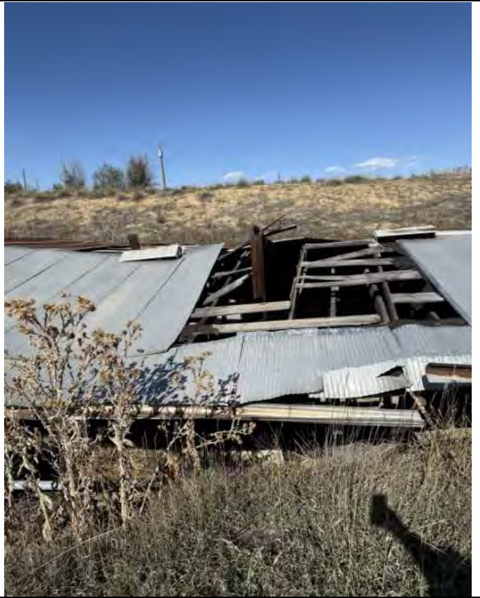
Description: Structure 6, center, area of slow active collapse
