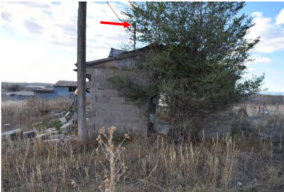
Figure 11. Wires entering on the north side of Outbuilding #2.
