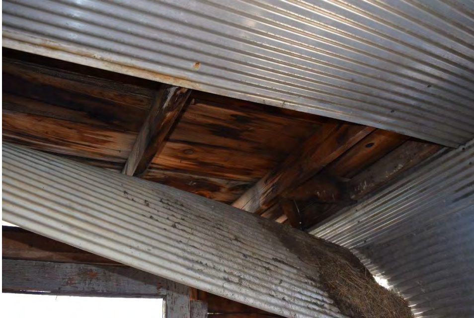
Figure 12. Structural members partially covered by interior finishes in the enclosed area of the Garage.
