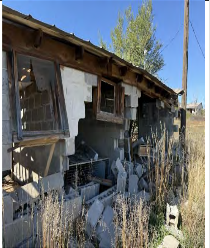
Description: Structure 7, NE corner that is collapsing, north view
