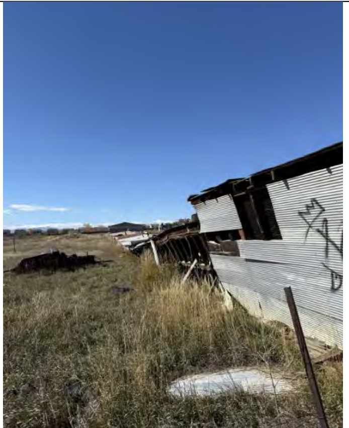
Description: Structure 6, east view, north side, visible lean to the structure
