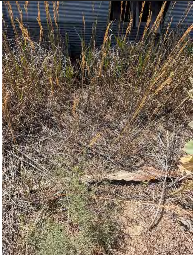
Description: Structure 6 Debris 9/9/25 Inspection
