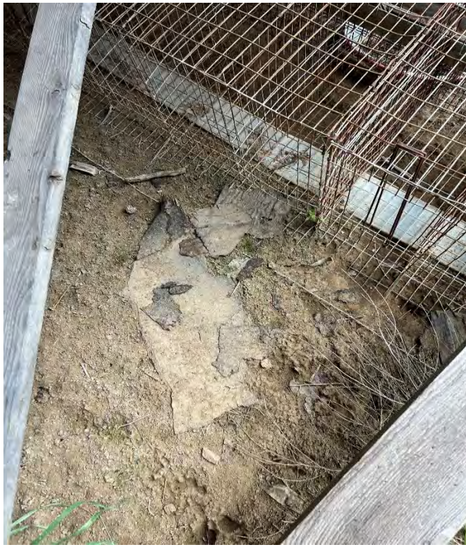
Description: Structure 6, ACM Roofing Tar Paper Debris 7/15/24 Inspection
