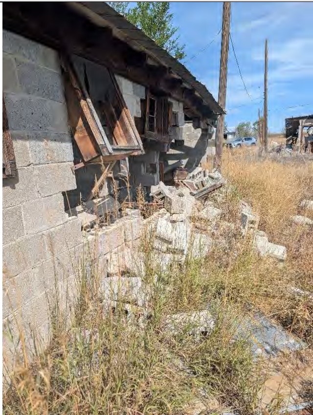
Description: Structure 7 Debris 9/9/25 Inspection
