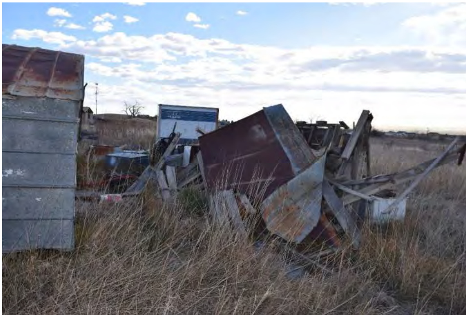
Figure 13. Collapsed portion of Outbuilding #3.
