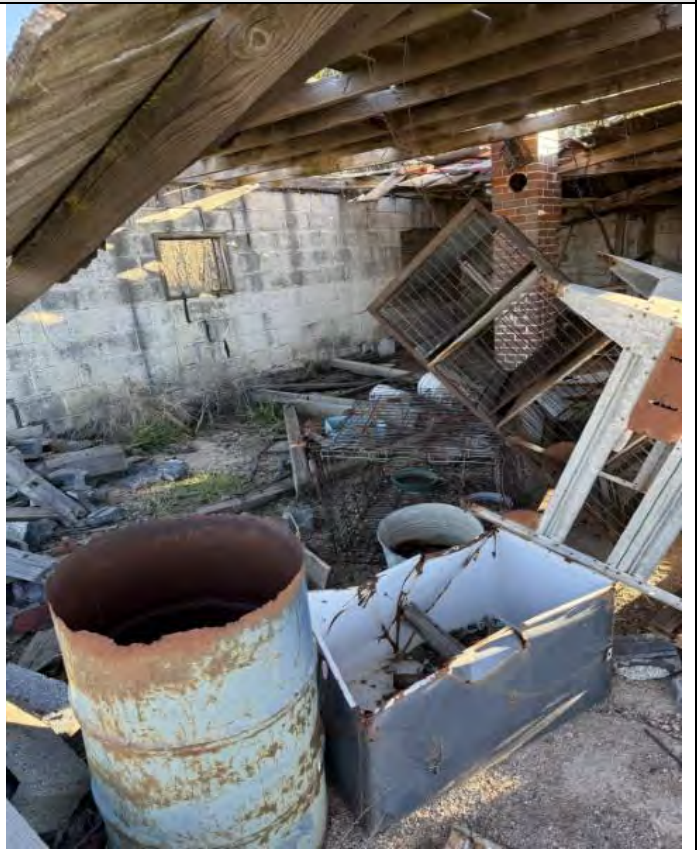
Description: Structure 5, west side collapse & debris
