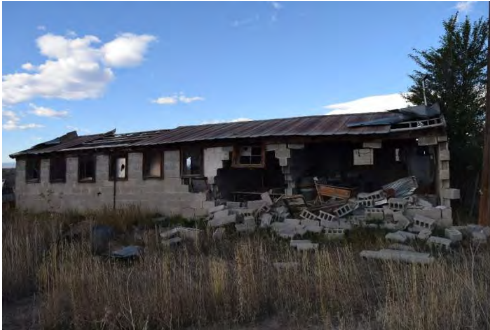
Figure 10. Collapsed north half of the east wall of Outbuilding #2.
