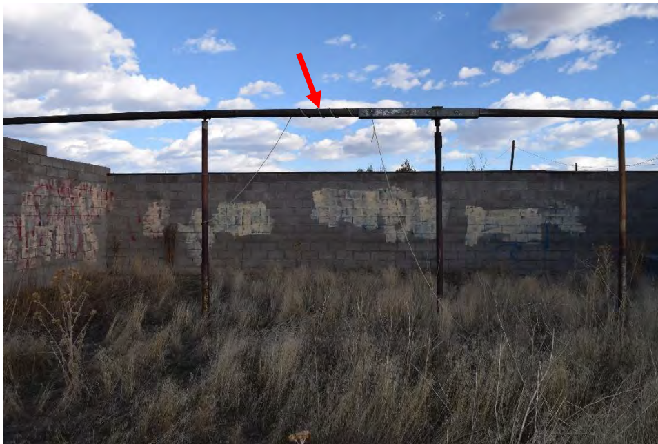
Figure 19. Wooden members spanning across intermittent steel tube columns on the south side of the CMU Wall Enclosure.
