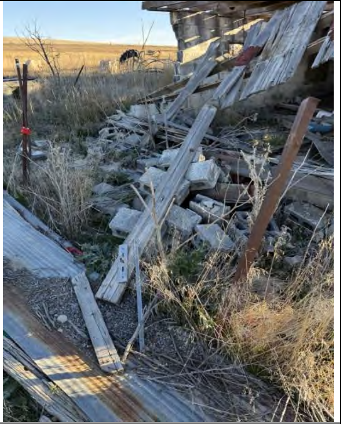
Description: Structure 5, west side collapse & debris
