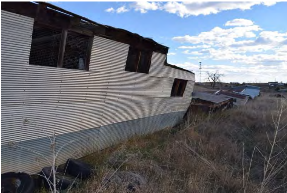
Figure 17. The south wall of the Hen House exhibiting a noticeable lean.
