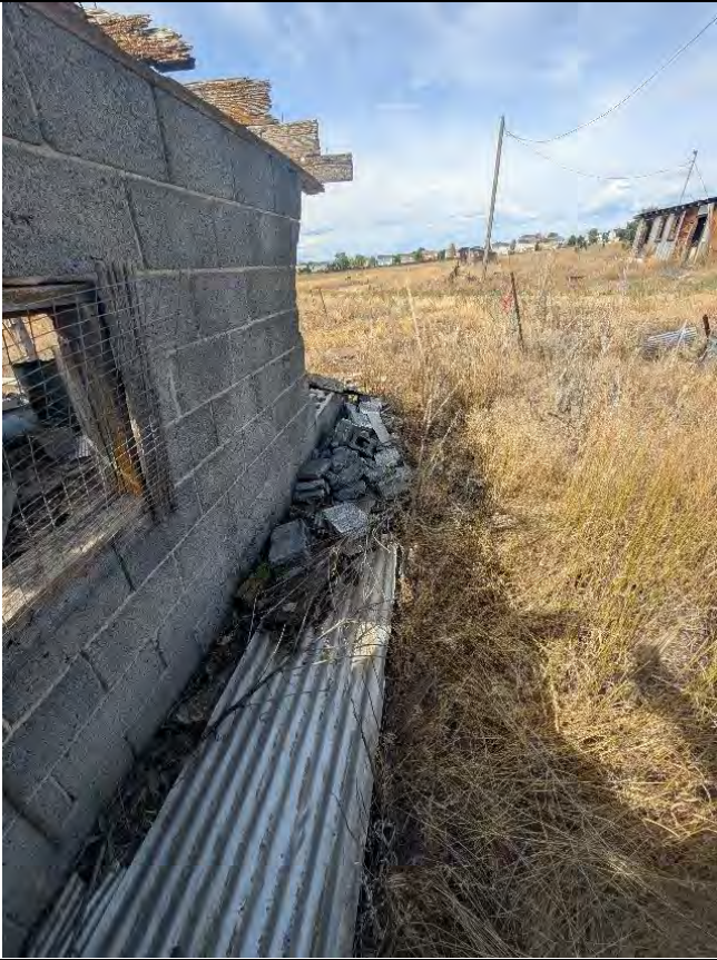
Description: Structure 5 Debris 9/9/25 Inspection
