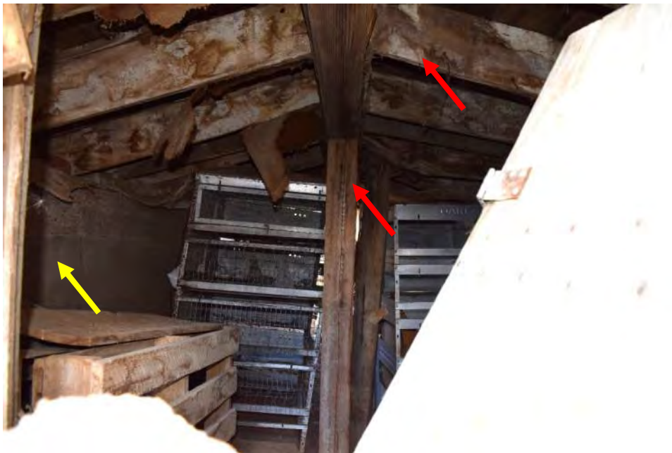
Figure 23. Dimensional lumber beams and columns (red arrows) and a concrete wall (yellow arrow) in the Cellar.
