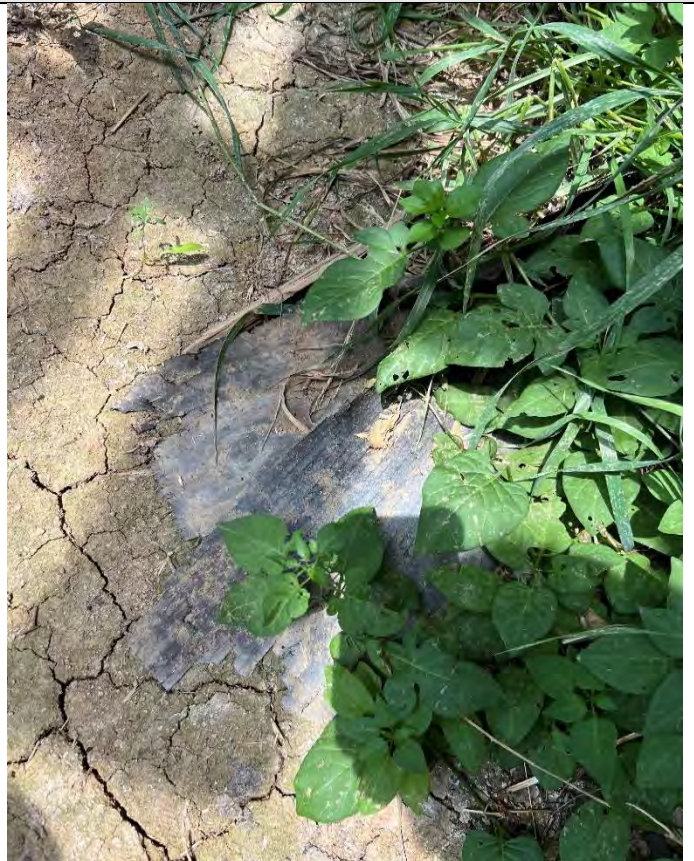
Description: Structure 6, ACM Roofing Tar Paper Debris 7/15/24 Inspection
