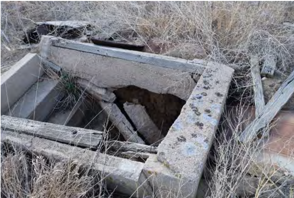
Figure 21. Broken concrete walls of the main entry of the Cellar.
