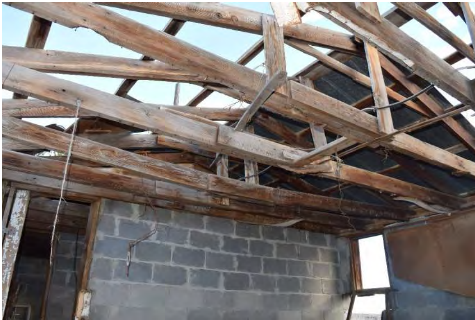
Figure 9. Wood roof trusses of Outbuilding #2 deflecting and showing signs of deterioration.
