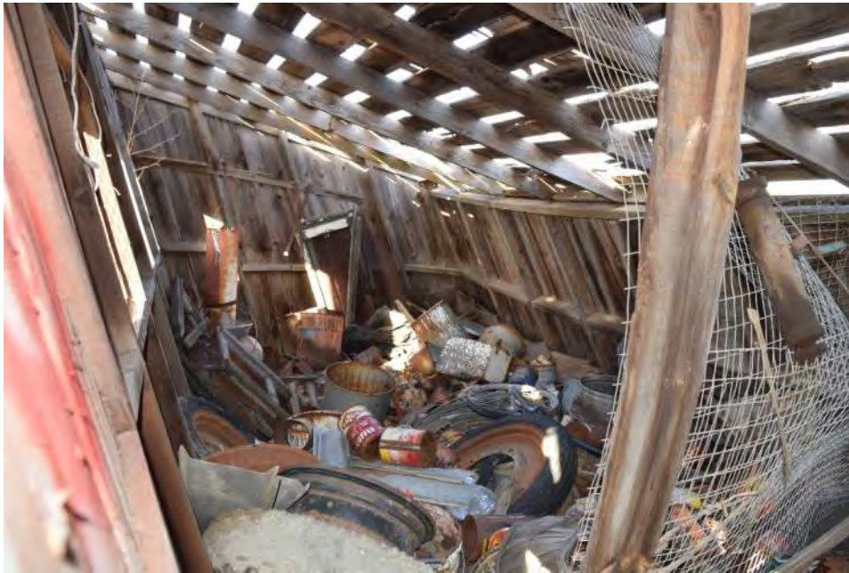
Figure 3. Interior view of the Chicken Coop showing a noticeable lean.
