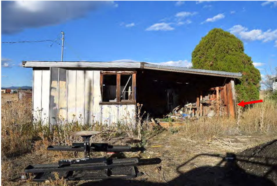
Figure 14. The northernmost wall of the Garage exhibiting a slight lean towards the south.
