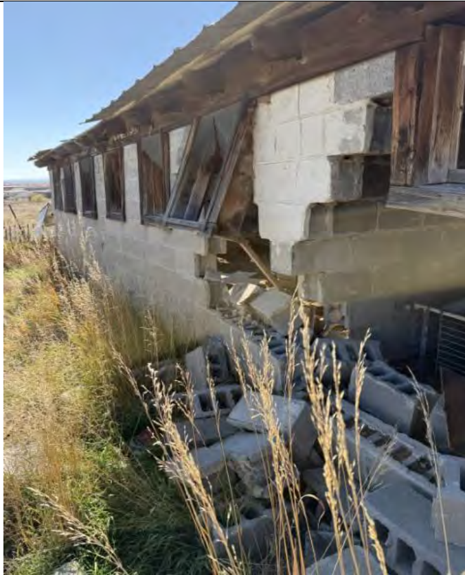
Description: Structure 7, NE corner that is collapsing, south view
