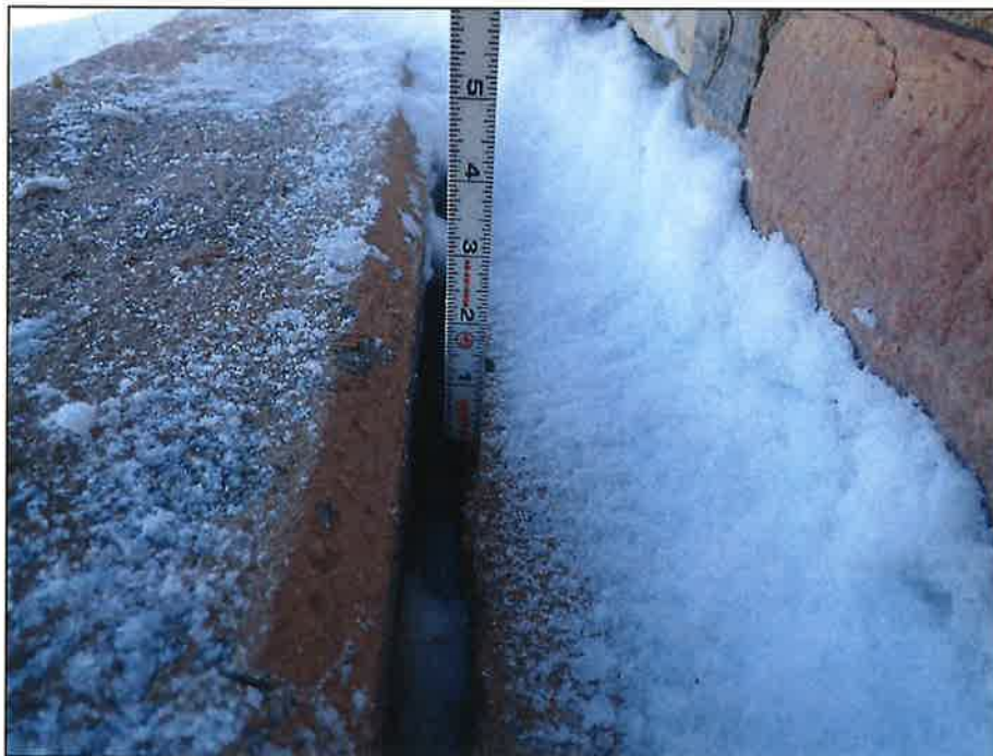
Typical Settled Approach Slab, Evident from the Differential Along the Edge of the Wingwalls at the Corners, Looking East
