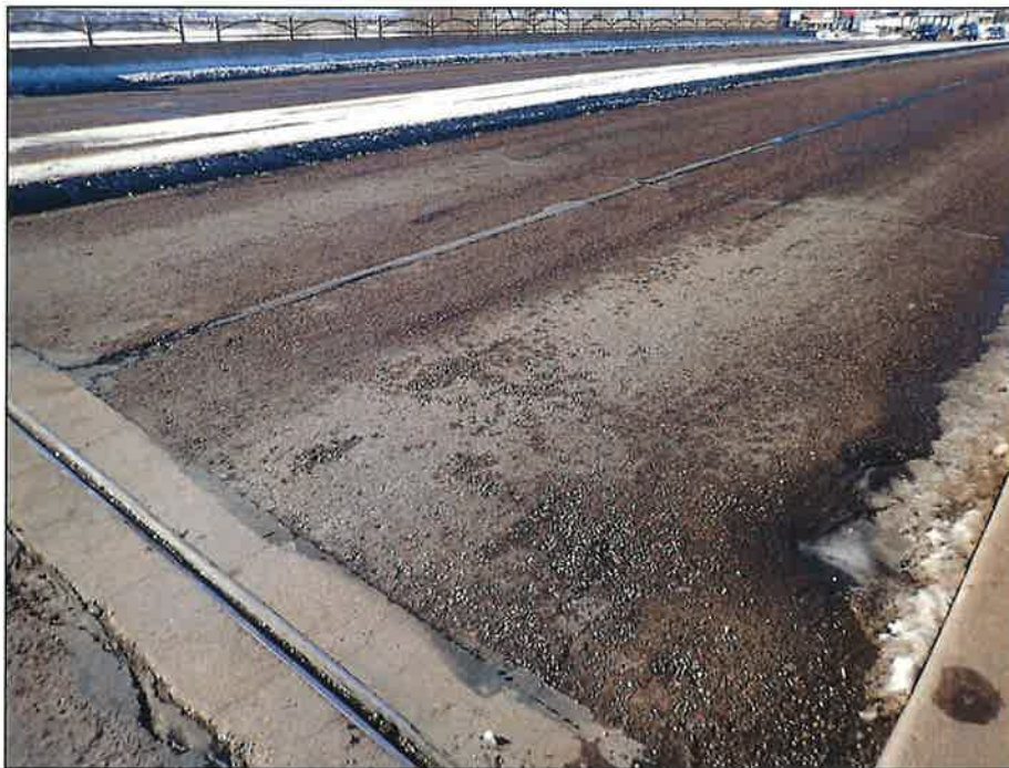
Typical Potholes Adjacent to the Sealed Gap in the Approach Slab Wearing Surfaces, Looking Northwest
