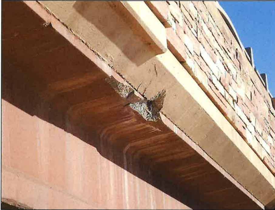
Spall with Exposed Rebar in the Exterior Top Flange of Girder 1O, 20 Feet West of Pier 2, Looking East
