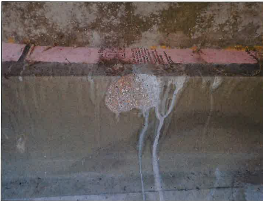
Spall in the Top Flange of Girder 1E at the West Abutment, Looking South
