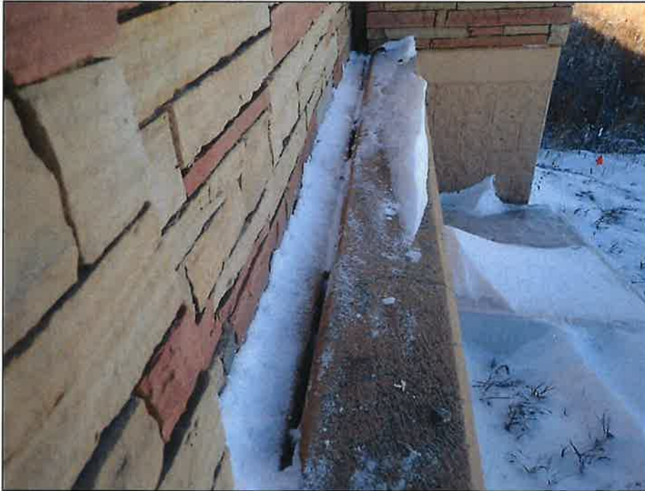
Typical Settled Approach Slab, Evident from the Differential Along the Edge of the Wingwalls at the Corners, Looking West
