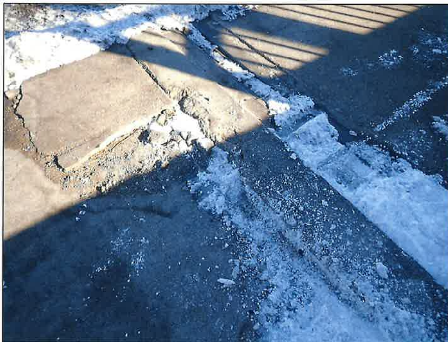
Missing Sidewalk Cover Plate and a 1.5 Inch Lip at the Southwest Corner, Looking East
