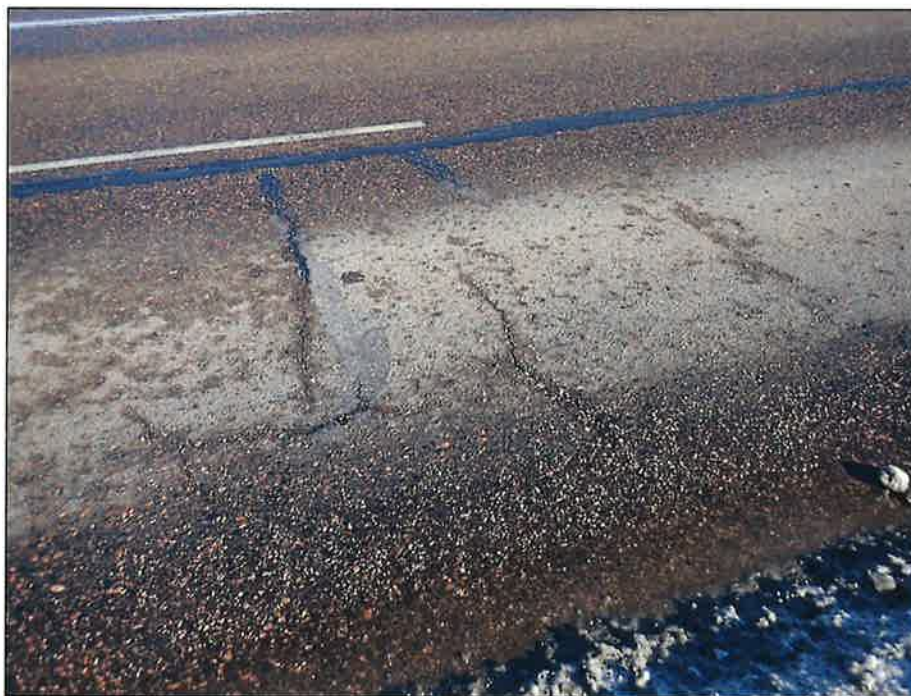
Typical Unsealed Cracks and Tar-Sealed Longitudinal Cracks in the Deck Asphalt Wearing Surface, Looking North
