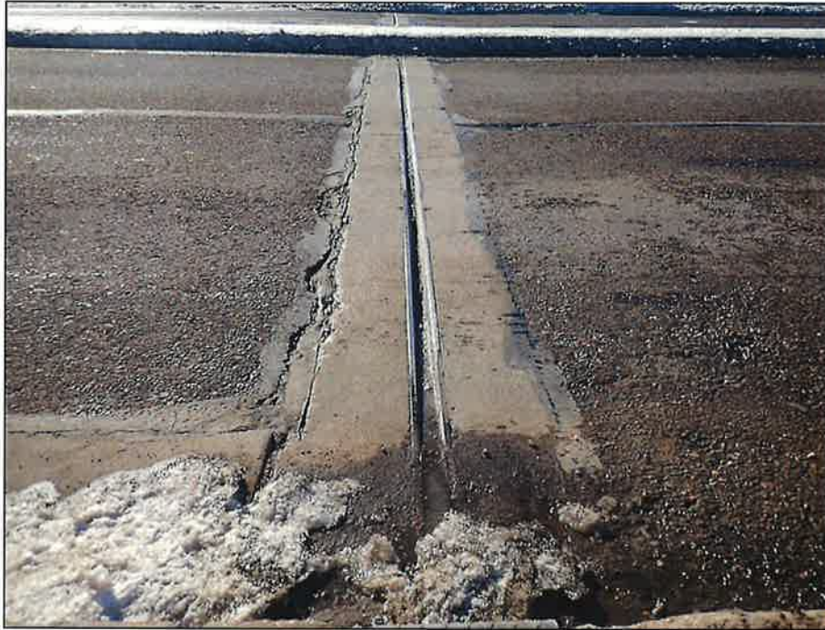
Typical Partial Loose Debris Impactation of the Strip Seal Expansion Joints, Looking South
