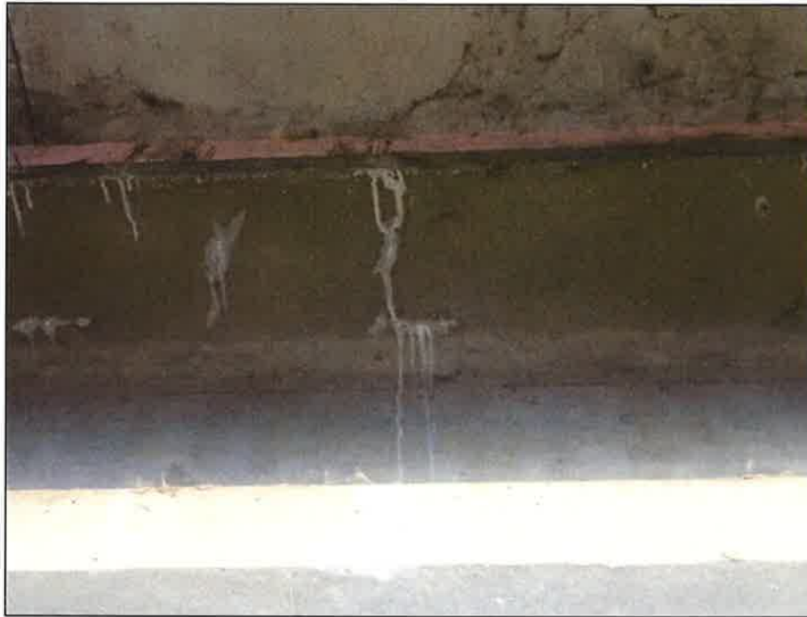
Typical Short Transverse Cracks with Efflorescence in the Underside of the Top Flanges of Several Girders, Looking South
