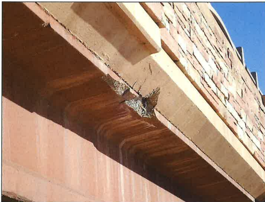
Spall with Exposed Rebar in the Exterior Top Flange of Girder 1O, 20 Feet West of Pier 2, Looking East
