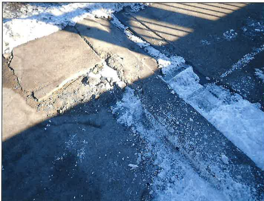
Missing Sidewalk Cover Plate and a 1.5 Inch Lip at the Southwest Corner, Looking East
