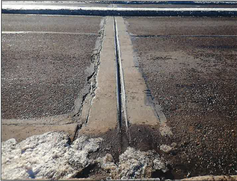
Typical Partial Loose Debris Impactation of the Strip Seal Expansion Joints, Looking South
