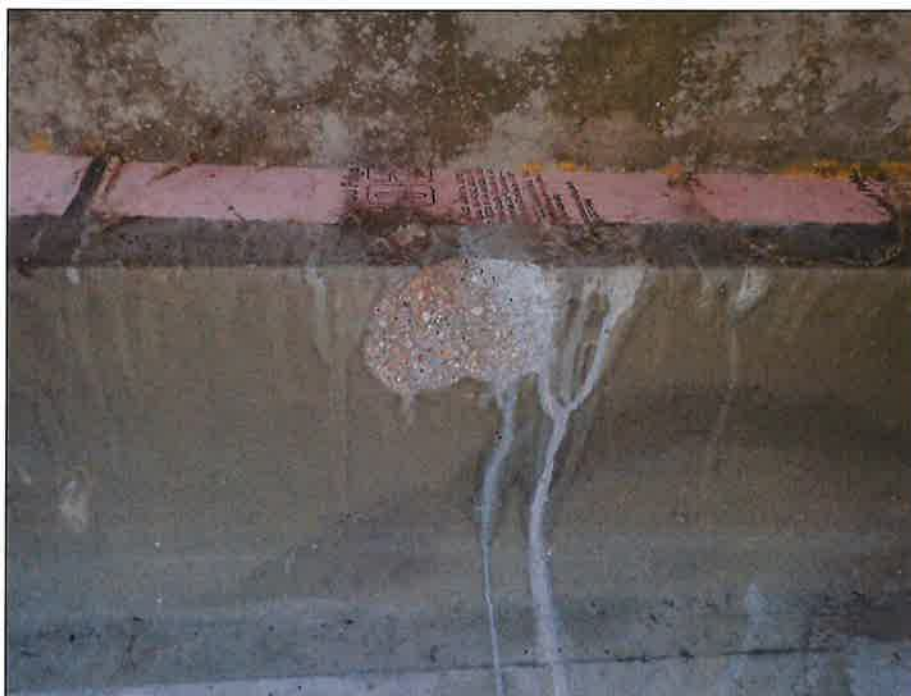
Spall in the Top Flange of Girder 1E at the West Abutment, Looking South
