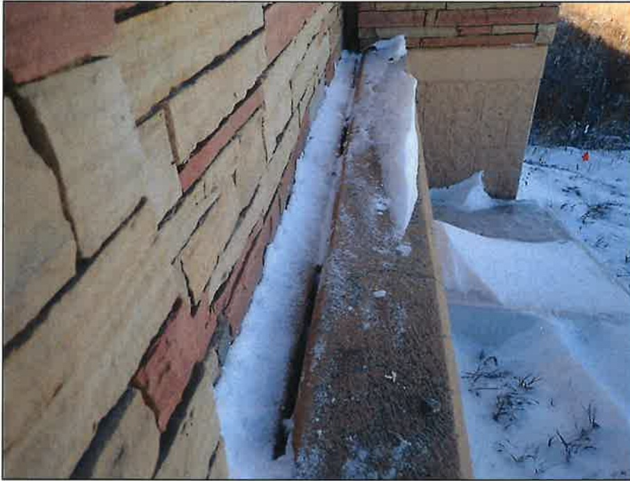
Typical Settled Approach Slab, Evident from the Differential Along the Edge of the Wingwalls at the Corners, Looking West
