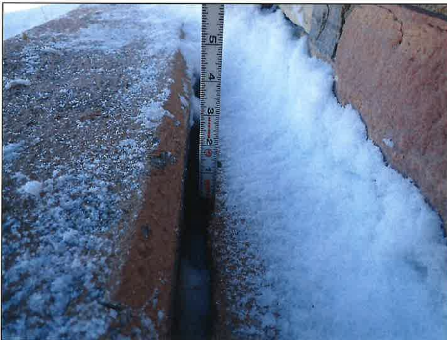
Typical Settled Approach Slab, Evident from the Differential Along the Edge of the Wingwalls at the Corners, Looking East
