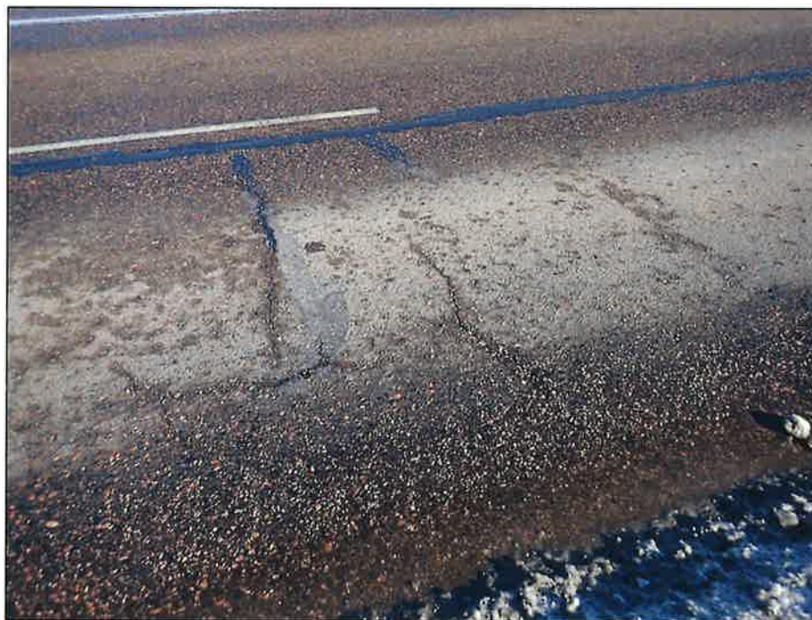
Typical Unsealed Cracks and Tar-Sealed Longitudinal Cracks in the Deck Asphalt Wearing Surface, Looking North
