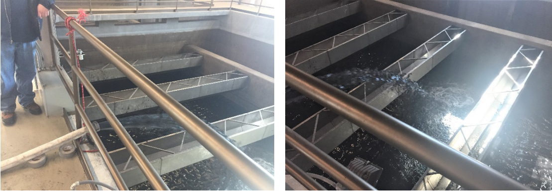
Figure 3 GAC Gravity Filters at Binney WPF, Aurora, CO
