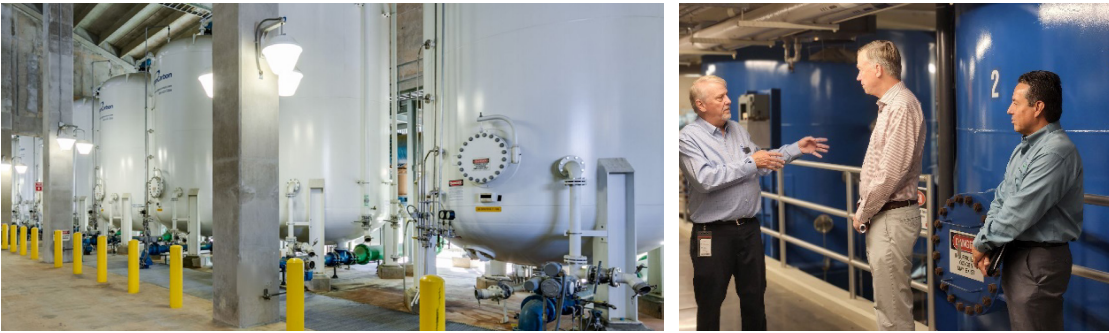
Figure 4 GAC Pressure Vessels at Wyckoff WTP, Marietta, GA (72 mgd) and Klein WTF, South Adams County, CO (14 mgd)
